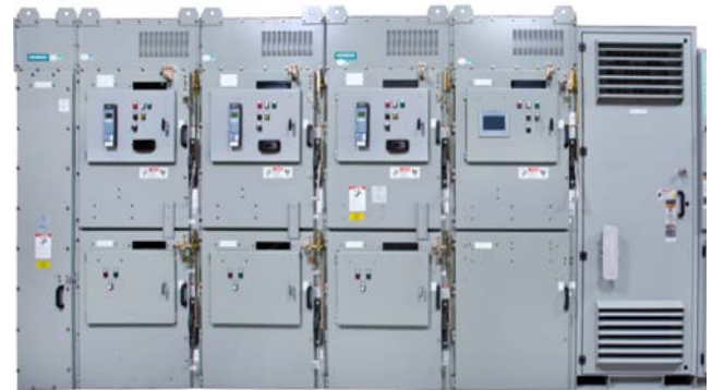
Figure 9: Switchgear and reactor lineup for 3 motor synchronous transfer application (for drive manufactured in the USA only)
