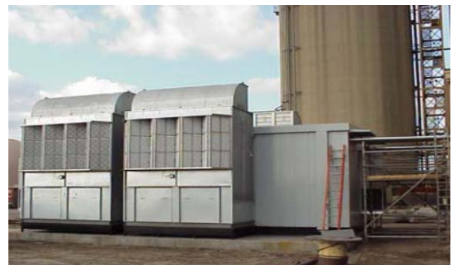
Figure 8 Installation with air-to-air heat exchangers and two drives in the building
